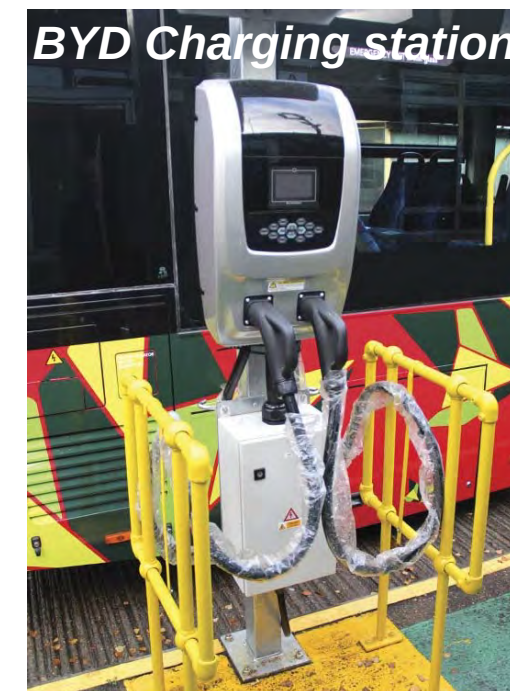
Photo 3.3 Station de recharge de BYD
